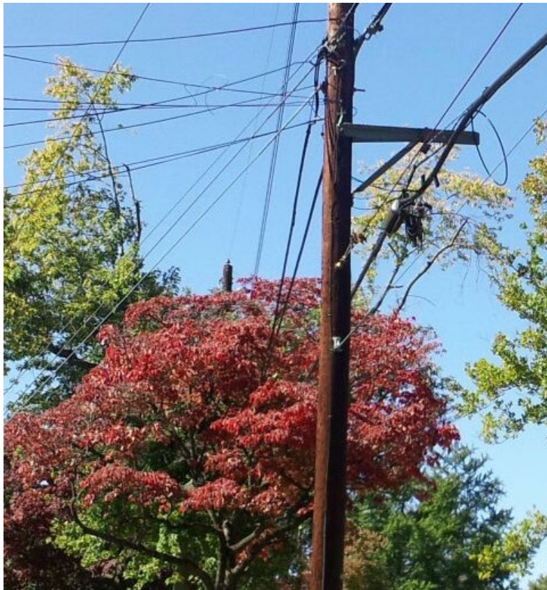
Figure 12: Example of extension arm on pole, enabling horizontal expansion of capacity
