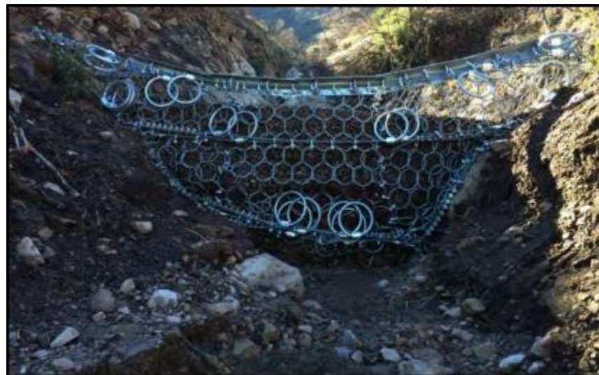
Figure 6-91 Debris Flow Barrier System
